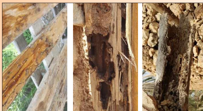
Figure 3. Heavy termite damage in commercial timber at Jazan, KSA.
